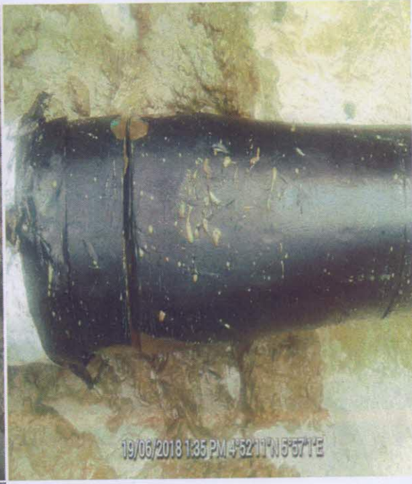
RUPTURED PART OF THE PIPELINE.
